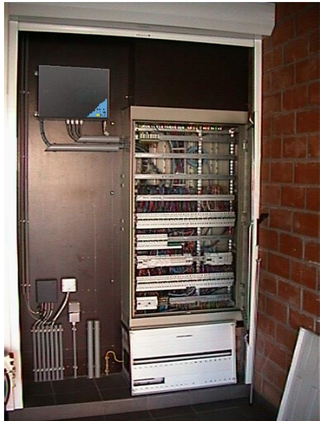
Figure 2: Clear division between input and output cables
